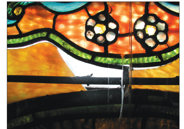
Photo courtesy of Doris Cultraro Broken glass with detached wire tie.
